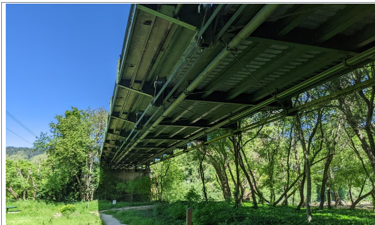
Photo 3 Looking northwest under the Guerneville Bridge at the existing force main hanging on the underside.
