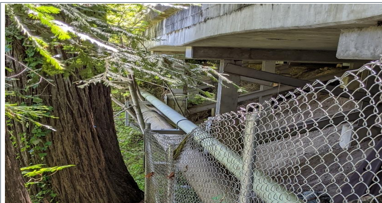
Photo 6 The existing 16-inch diameter CMLC steel force main and 8-inch diameter gravity sanitary sewer suspended along the Hwy 116 viaduct.
